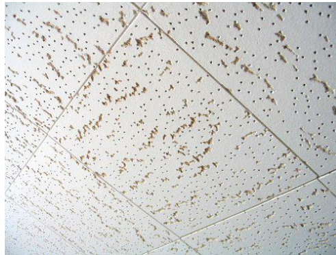
Asbestos containing ceiling tiles
