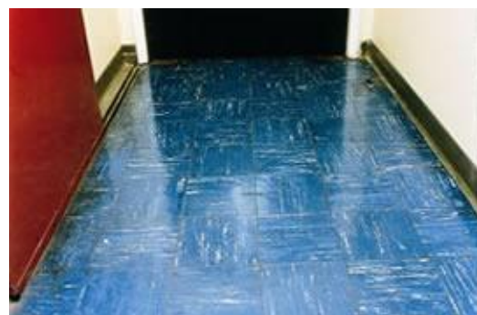
Asbestos containing floor tiles in a corridor
